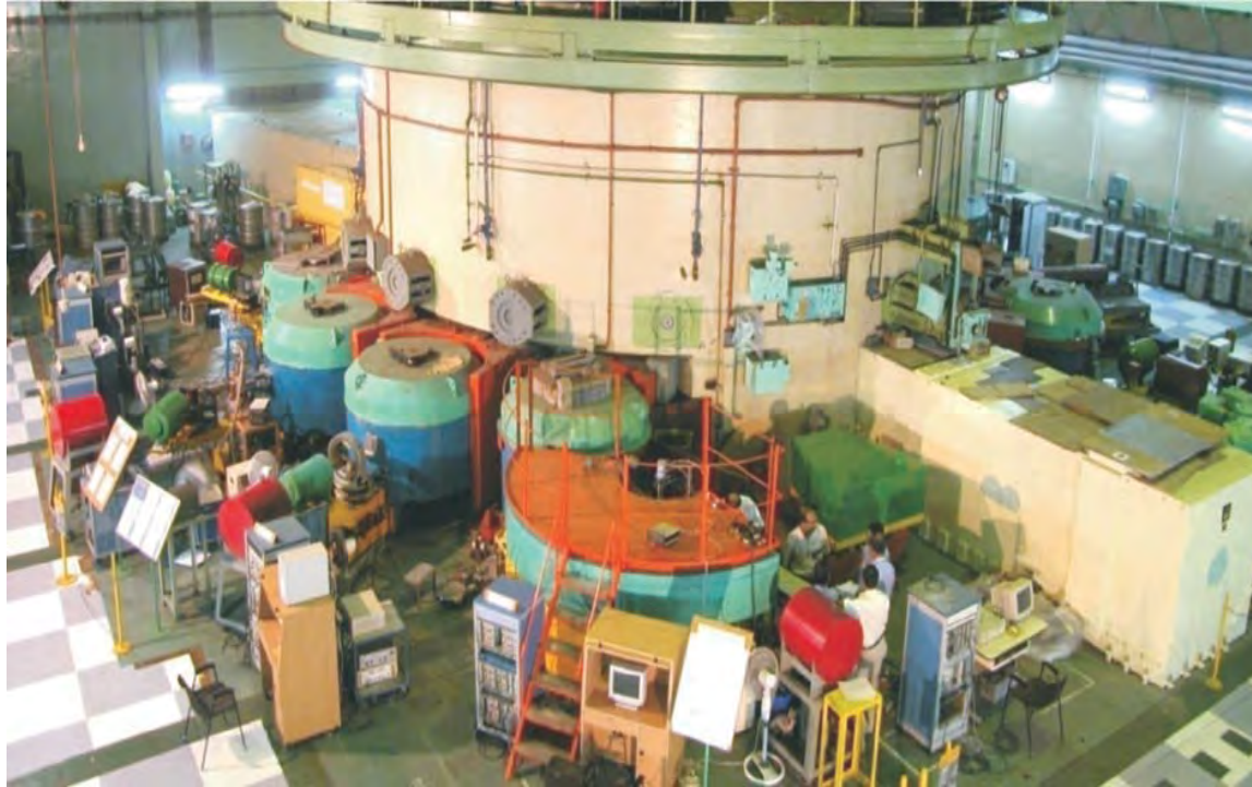
Neutron Scattering Facilities inside Dhruva Reactor Hall
